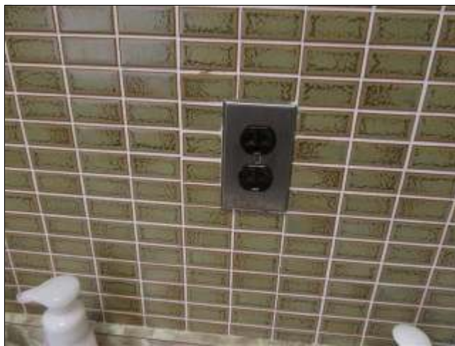
7.4 Item 2(Picture) Not GFCI protected/Typical.
