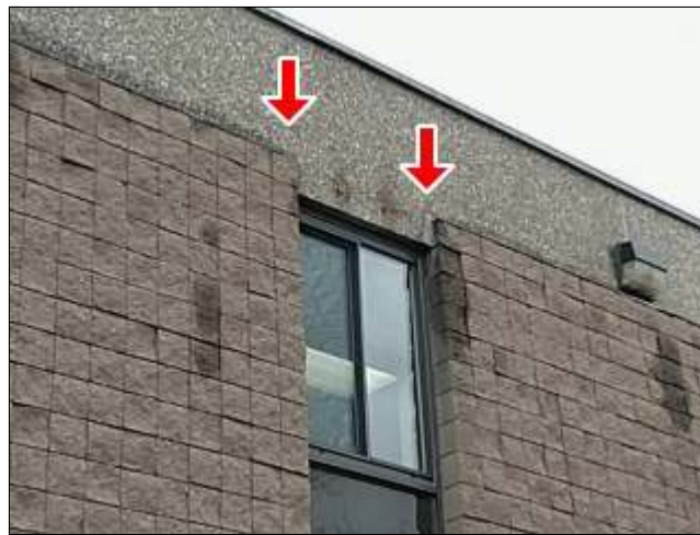
4.0 Item 4(Picture) Poor flashing detail.
