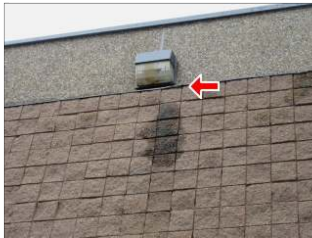
4.0 Item 6(Picture) Seam in flashing under light.
