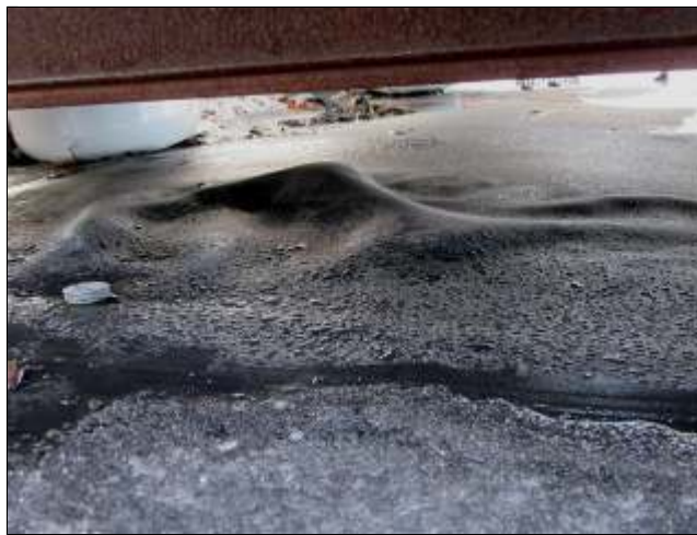
3.0 Item 2(Picture) Membrane under chiller.
