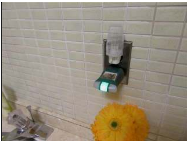
7.4 Item 3(Picture) Not GFCI protected.
