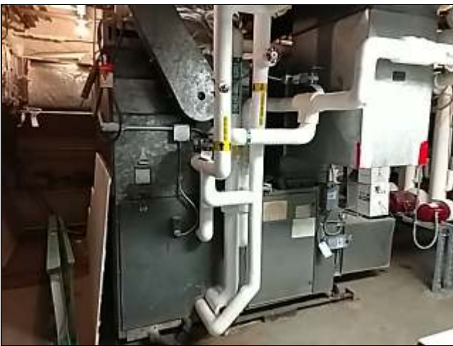
8.0 Item 3(Picture) Air Handlers in good condition.
