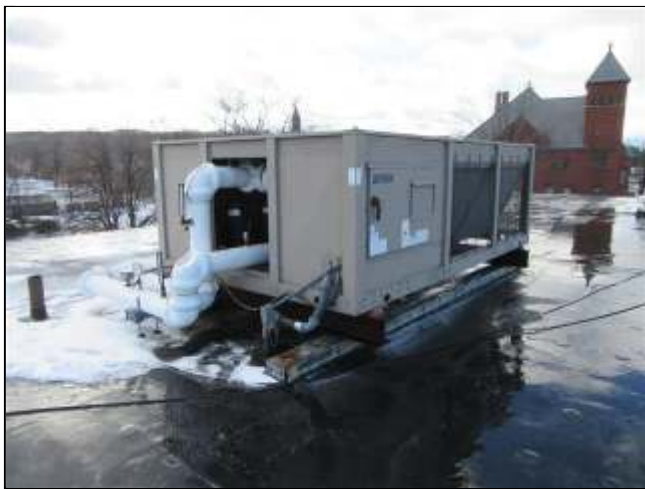
8.5 Item 1(Picture) Chiller on roof.
