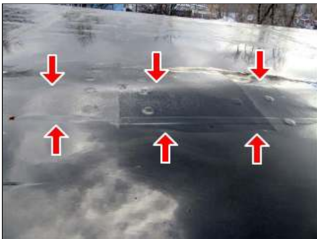
3.0 Item 5(Picture) Underlayment heaving.
