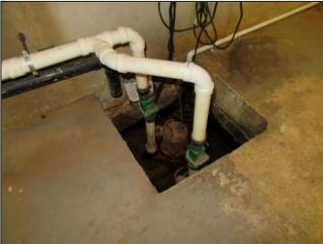
6.4 Item 1(Picture) Sump pump.
