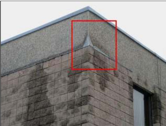
4.0 Item 13(Picture) Previous repair.
