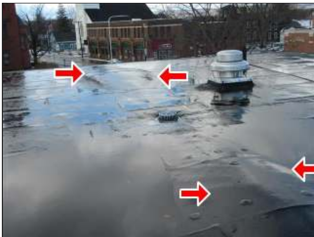
3.0 Item 3(Picture) Underlayment heaving.
