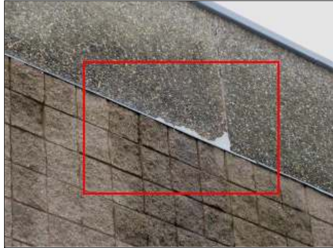
4.0 Item 12(Picture) Previous repair.
