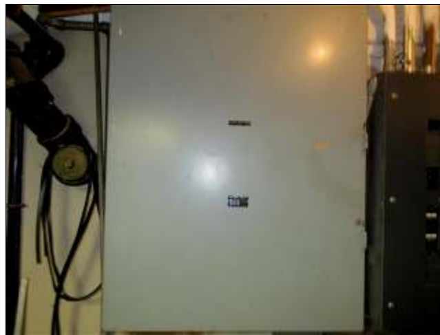
2.1 Item 2(Picture) 1200 AMP main disconnect.
