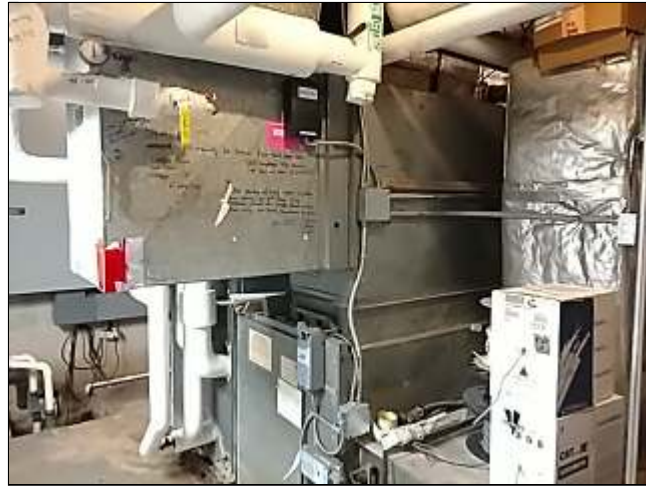
8.0 Item 2(Picture) Air Handlers / secondary
