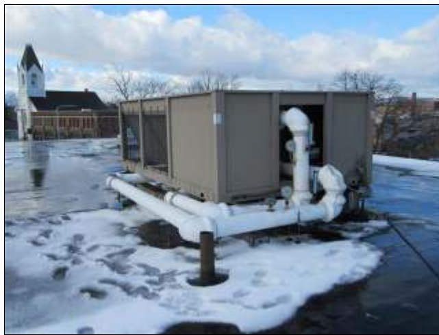
8.5 Item 2(Picture) Chiller/MFG 2009.
