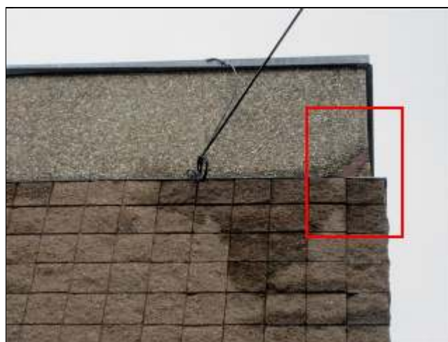
4.0 Item 8(Picture) Previous repair.
