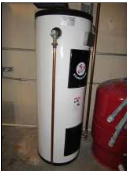
6.2 Item 1(Picture) MFG 2012/installed 2014.
