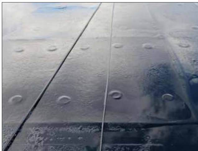
3.0 Item 6(Picture) Fasteners pressing against membrane.
