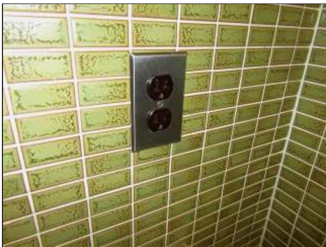
7.4 Item 1(Picture) Not GFCI protected.
