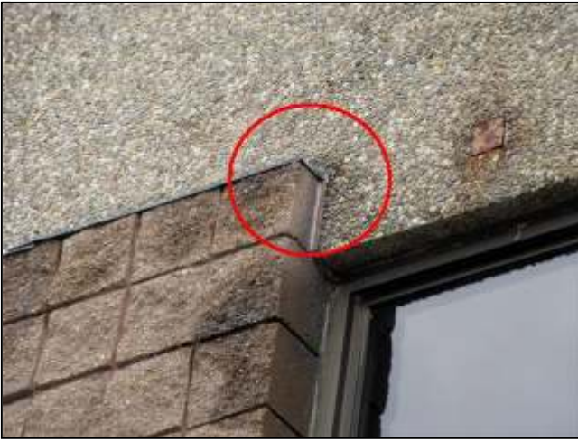
4.0 Item 9(Picture) Poor flashing detail.
