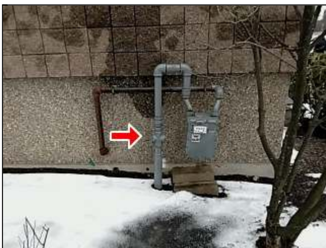
2.2 Item 1(Picture) Gas meter located at right rear building.
