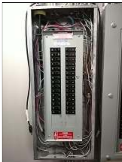
7.1 Item 5(Picture) View inside 200 AMP/2ND floor.
