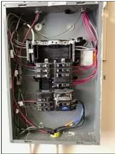
7.1 Item 6(Picture) View inside 60 AMP/1ST floor.
