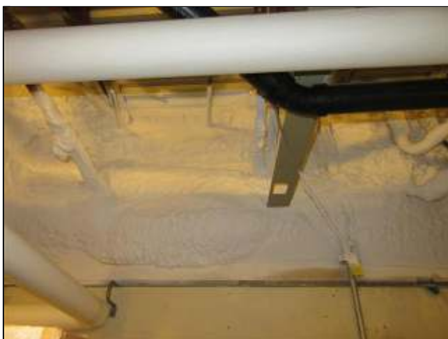
5.4 Item 1(Picture) Spray foam at perimeter/typical.
