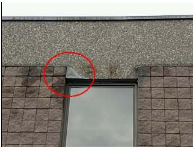
4.0 Item 3(Picture) Previous repair.
