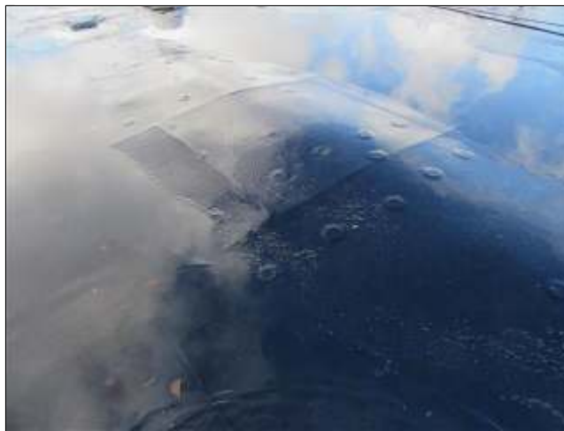
3.0 Item 4(Picture) Underlayment heaving.
