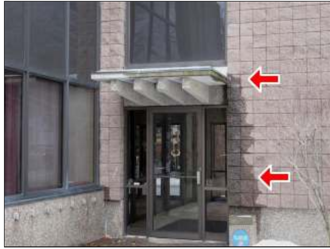
4.0 Item 10(Picture) Poor flashing detail.
