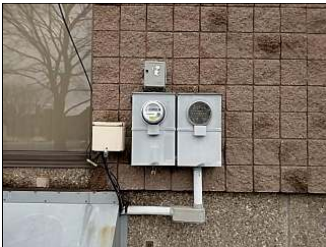
2.1 Item 1(Picture) Single meter located at rear building.
