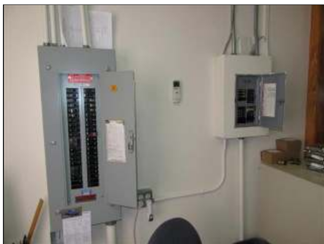
7.1 Item 3(Picture) 1ST floor panels.
