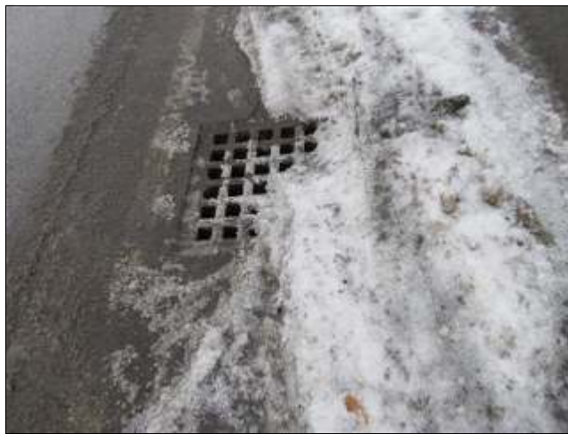
1.1 Item 2(Picture) Drain blocked.
