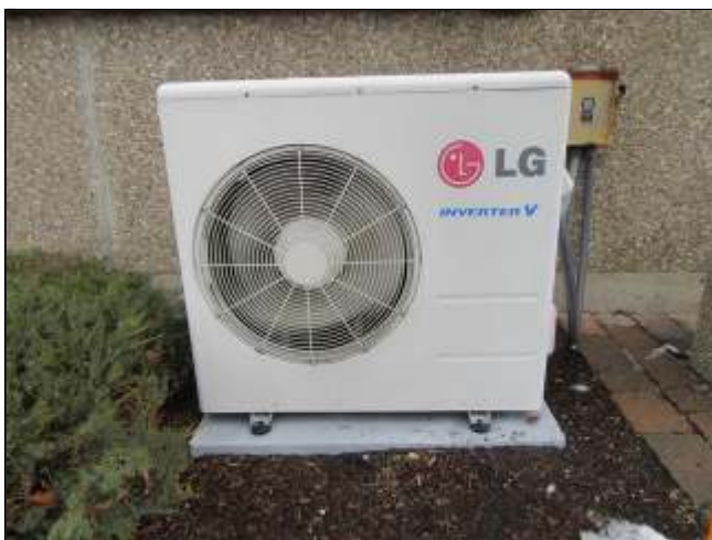
8.5 Item 3(Picture) Mini split for IT room/MFG 2000.
