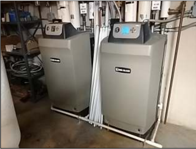
8.0 Item 1(Picture) 1st and 2nd floor primary boilers.
