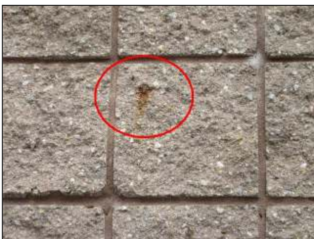
4.0 Item 7(Picture) Evidence of moisture behind veneer.
