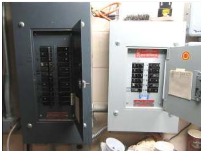
7.1 Item 2(Picture) Basement service panels.
